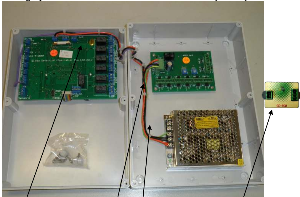
Photograph shows standard 2400 with NO VSD drive (GD690)
